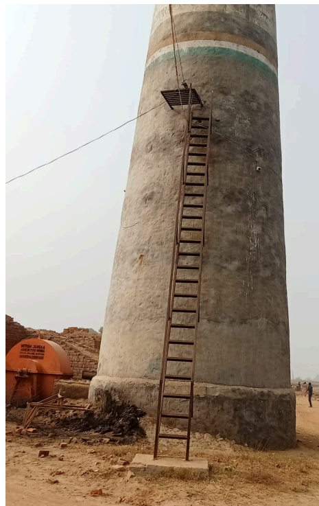
Non-Operational Bhatti, Ladder, Gravitational Settling platform
